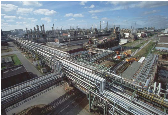
Figure 1-1 Pipes at Marl Chemical Park
