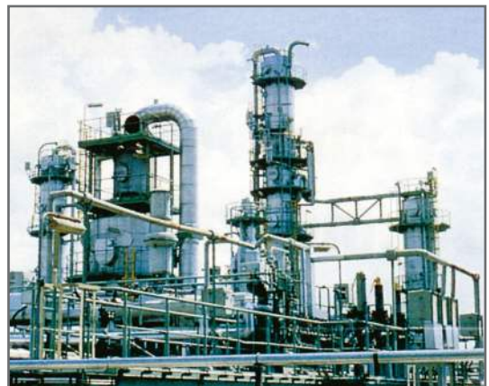
Figure 1: Industrial chemical plant
