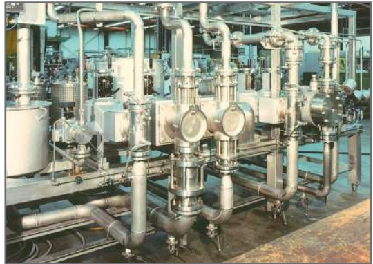
Figure 1: Pipelines in a chemical plant
